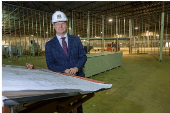
United Way of Southwest Virginia President and CEO Travis Staton is overseeing the $25 million transformation of a former Kmart in Abingdon into a regional child care and workforce development hub. Photo by Earl Neikirk
