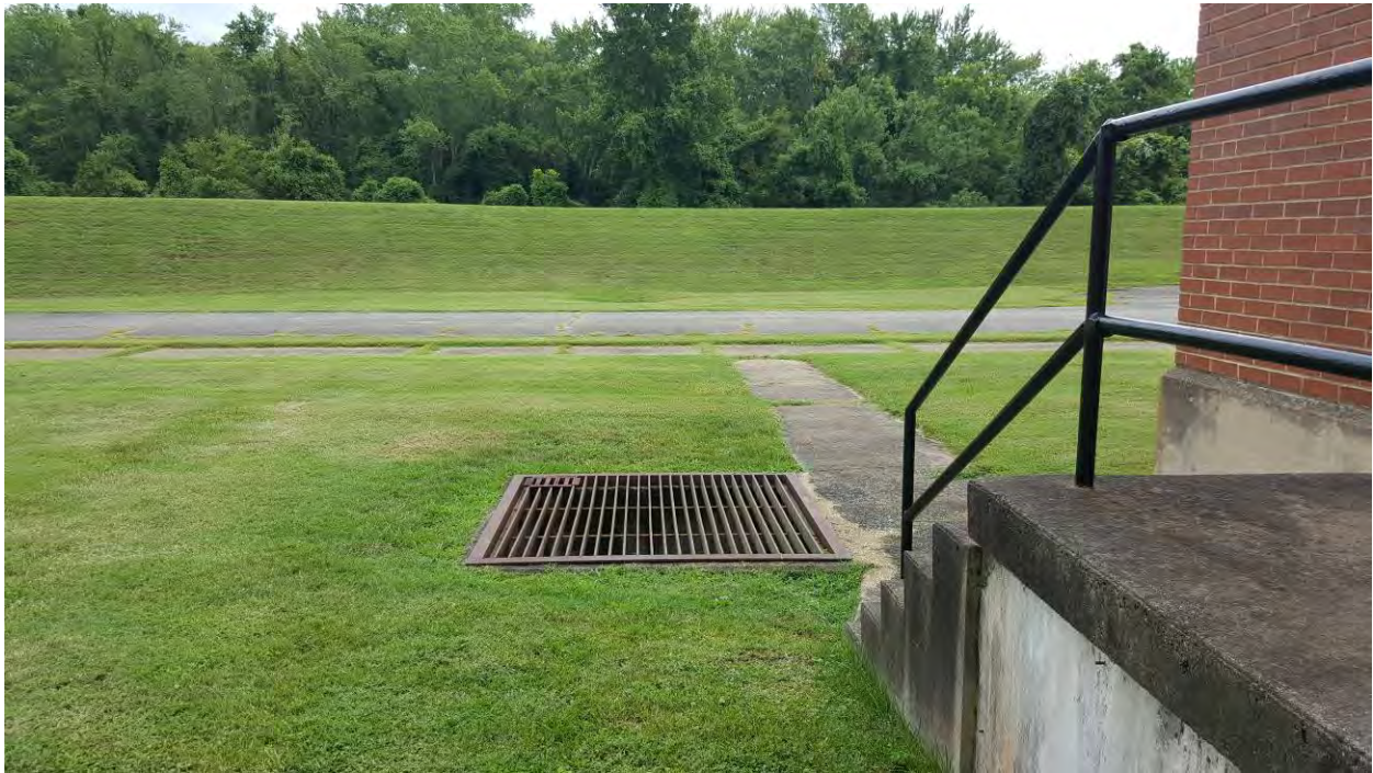
Image 1. View of drainage inlet from southeastern face of building with berm in the background.
