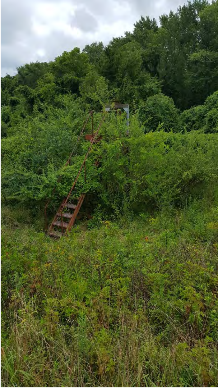
Image 3. Sluice gate valve at northern-most outfall.
