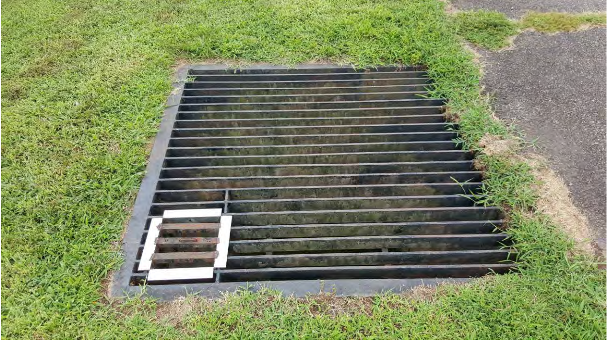
Image 4. Drainage inlet with access hatch for portable pump suction line.
