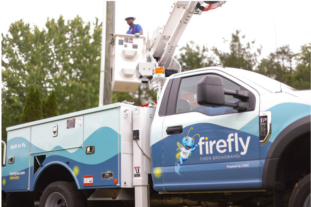
Firefly installer operates a bucket truck in rural Nelson County. Photo credit: Firefly Fiber Broadband SM
